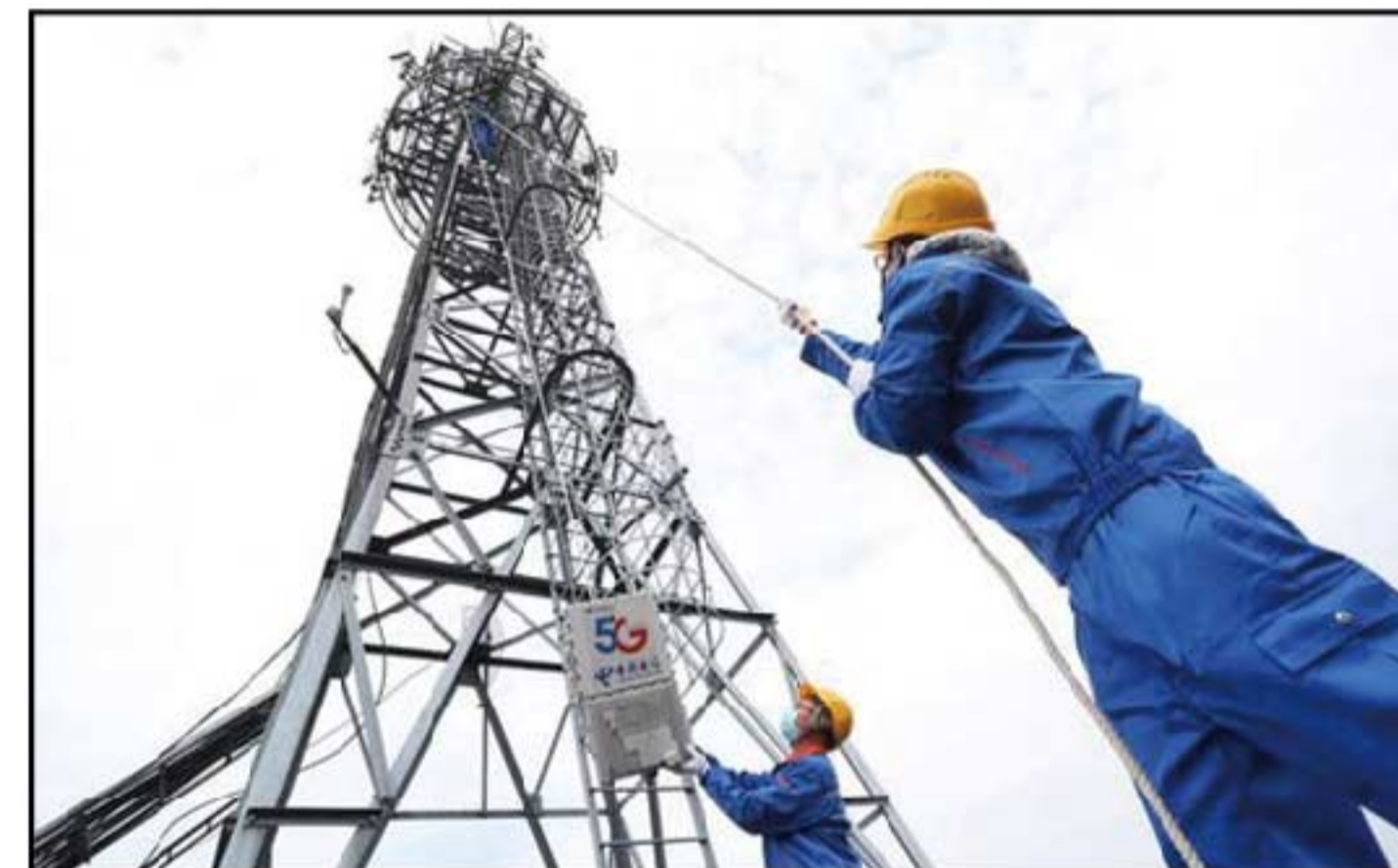
Telecom base station
