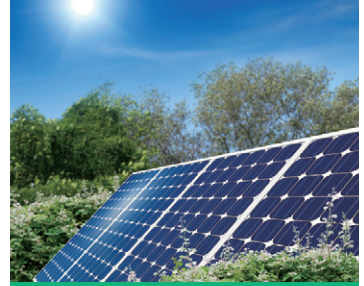
Solar power system
